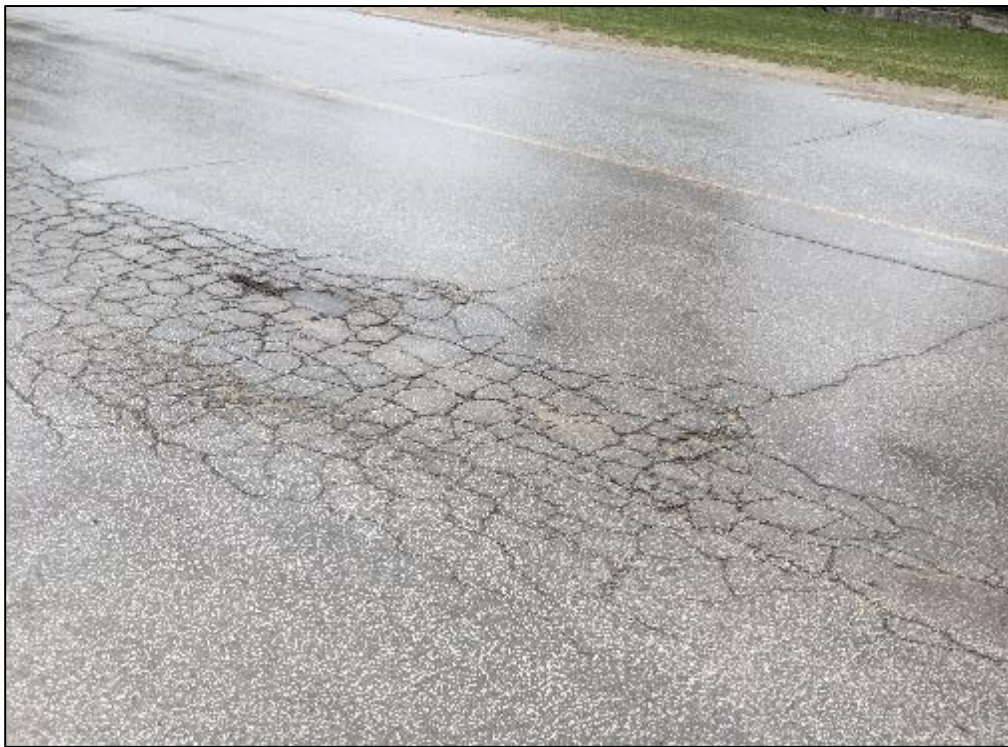
Figure 3: Example of poor pavement conditions on No 2 Side Road (TNS, 2021).
