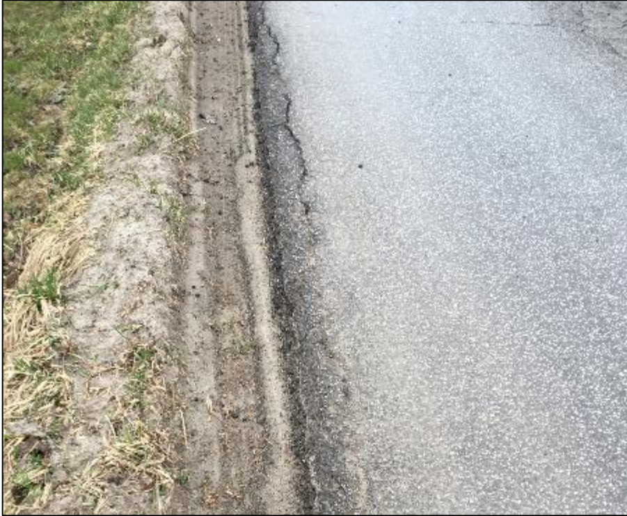
Figure 4: Example of pavement edge drop-off conditions on No 2 Side Road (TNS, 2021).
