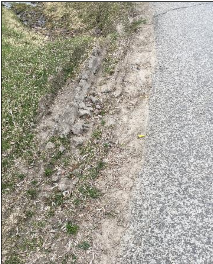
Figure 7: Tire tracks on the shoulder at the northeast corner of the existing truck access and No 2 Side Road location (TNS, 2021).
